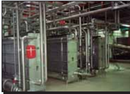
Pressure transmitter on line
