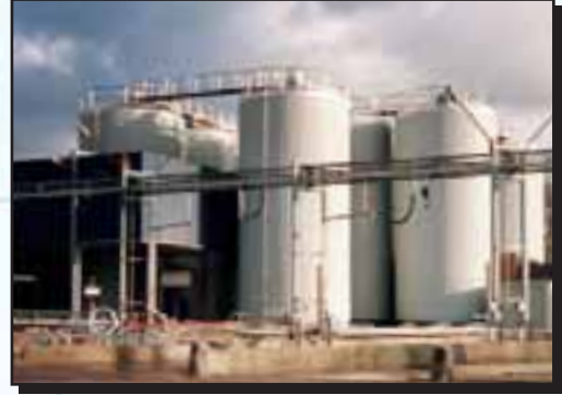
Level measurement on storage tanks
